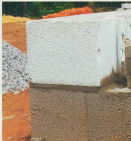
The tie that binds. Anchor bolts set in the concrete footing are attached to threaded rod running through the walls. Access is provided by a U-shaped cutout.
