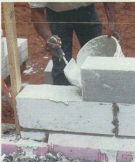
Mortar joints must be exact. A special trowel helps to ensure precise mortar thickness for block walls. Joints are flush with the wall.
